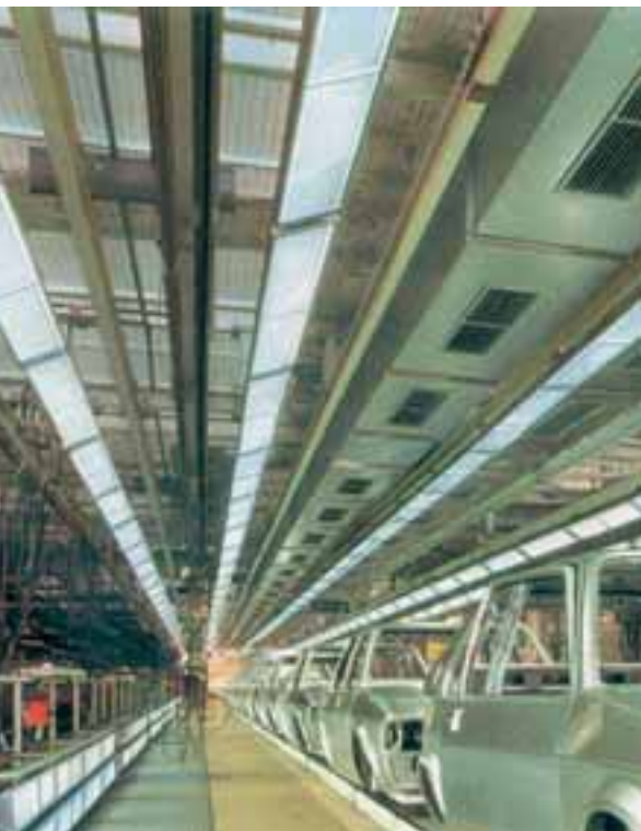
Intensive but glare free lighting with parabolic louvers in factories
